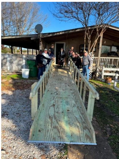
Compatriot Mike Tull assisted building a wheelchair ramp for a veteran here in Waxahachie (7 people and about 4 hours each to build and install).
